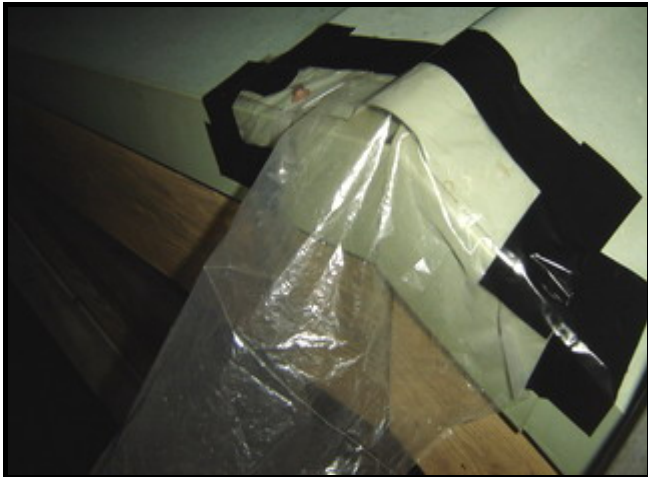
Fig. 6. Exclusion of the bats from the main entry point in the roof capping.
